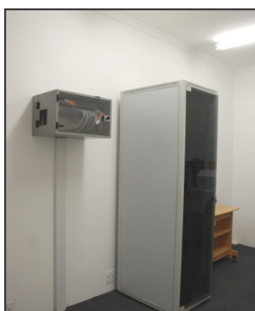
Computer server room plastered with Pratliperl to reduce energy requirements for cooling.
